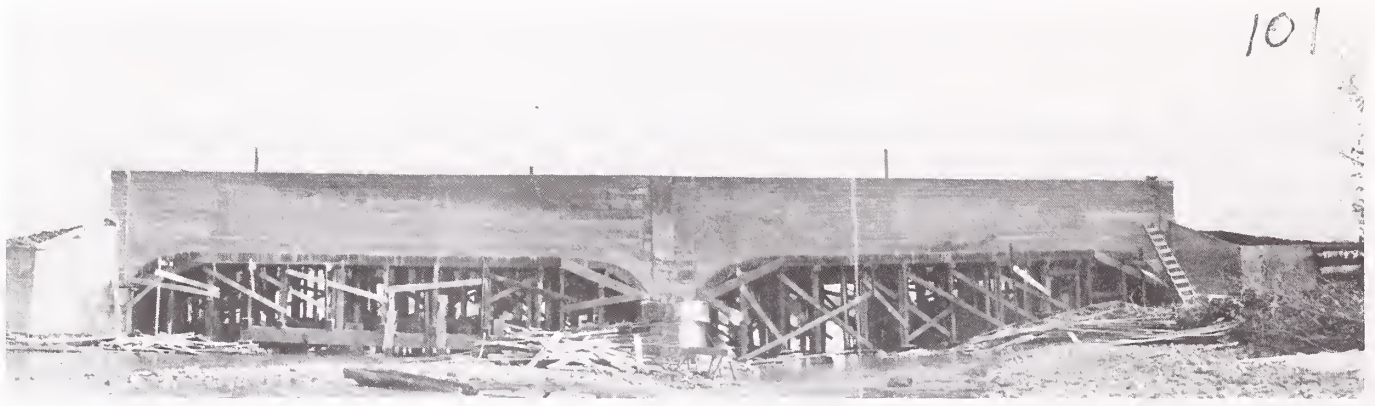
The completed bridge after the forms had been removed. The forms underneath the bridge were left in place until the concrete had cured (Montana Historical Society).
